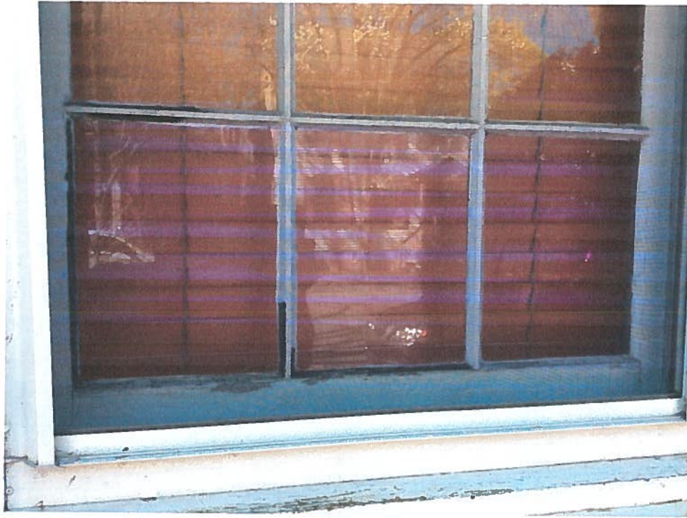
Figure 6. Deteriorating windows at 54 E Wall St – front of house
