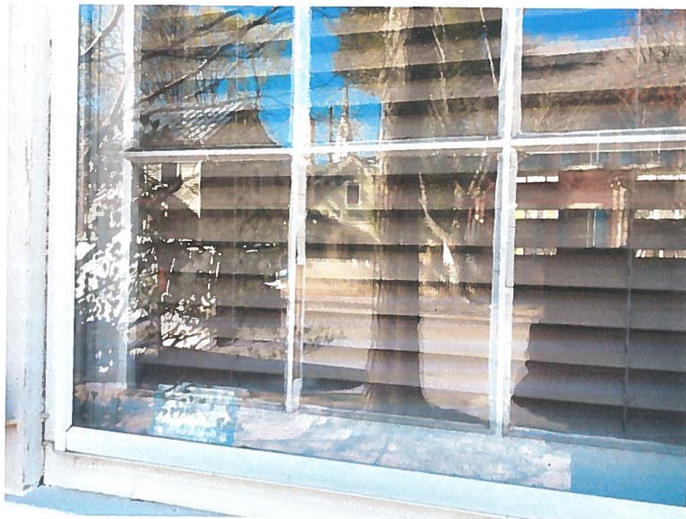
Figure 7. Deteriorating windows at 54 E Wall St – front of house
