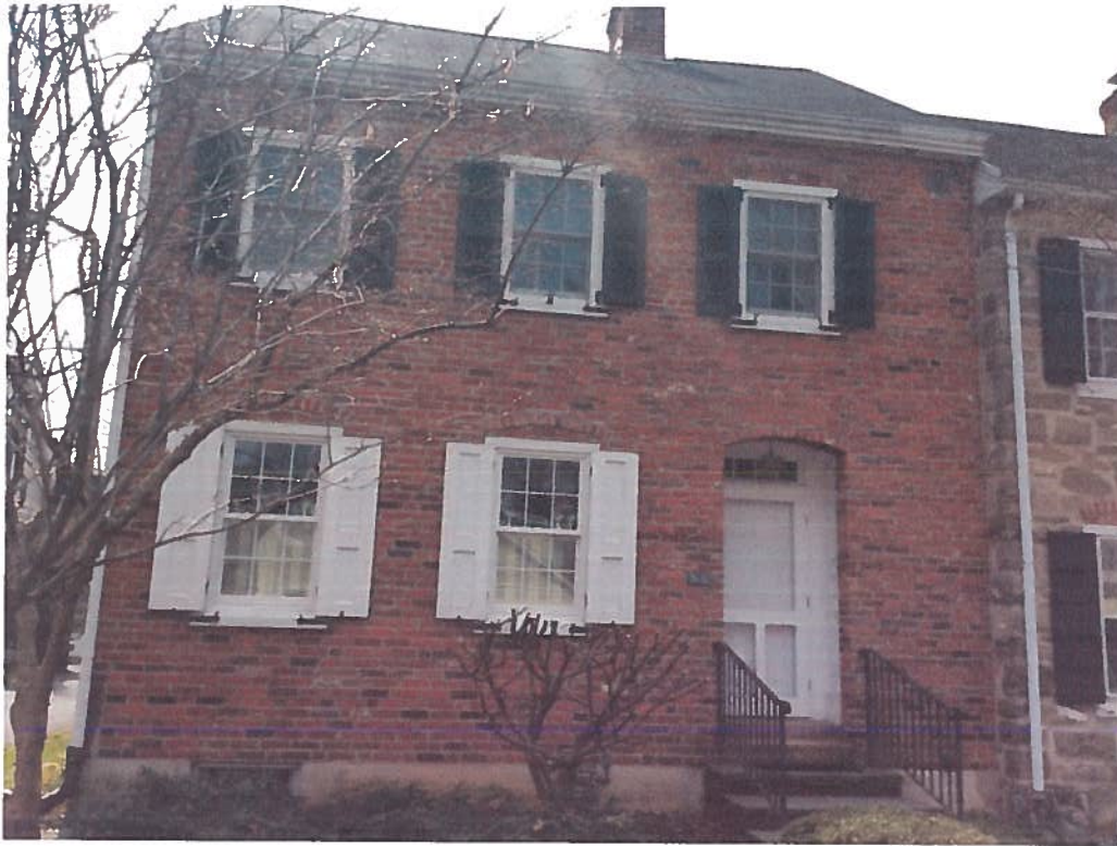
Figure 8. Recently installed Anderson Woodright Series 400 windows at 54 E Wall St –front of house
