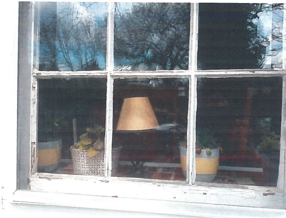
Figure 3. Deteriorating windows at 54 E Wall St – rear of house
