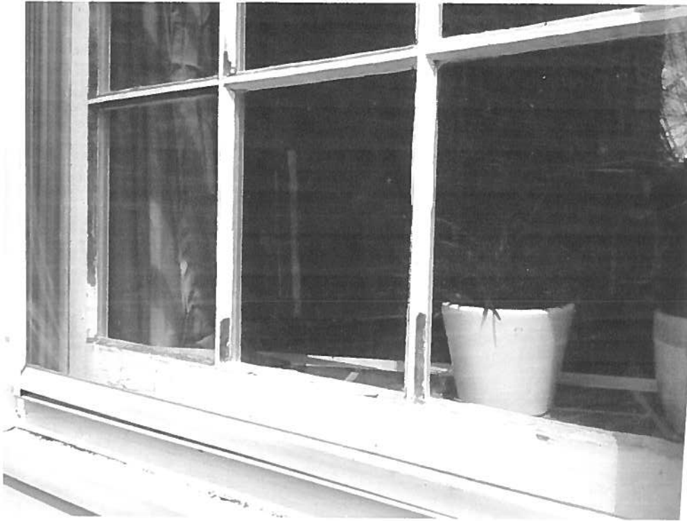
Figure 4. Deteriorating windows at 54 E Wall St – rear of house
